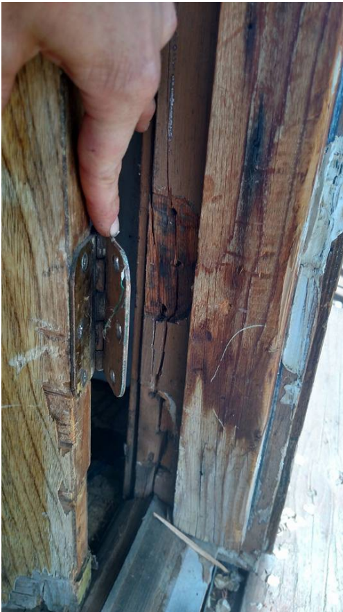
They fixed the crack in the frame for the front door by gluing it.
