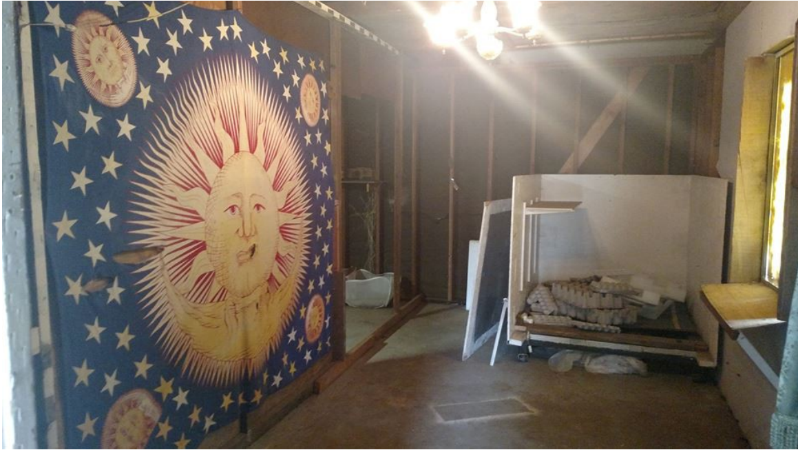
This was being built into a recording studio, & was further along this this at the time of the couples' removal. Ms. Wilson has written around 40 original songs & this would have been her first time being able to record albums.
