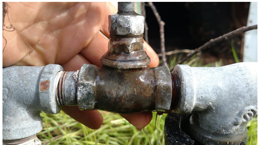
The main line to the water supply BEFORE the couple mended it.
